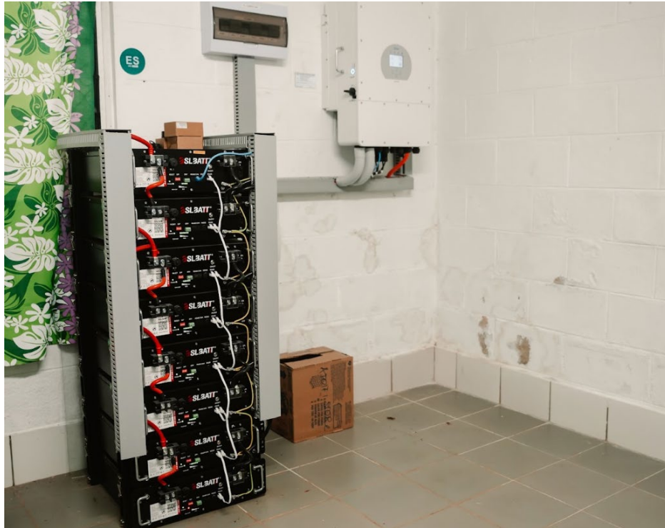
Caption 1: The Atoifi College of Nursing's main administration building, which includes two classrooms, a library, computer laboratory, and clinical laboratory, now has a reliable and clean supply of electricity.
